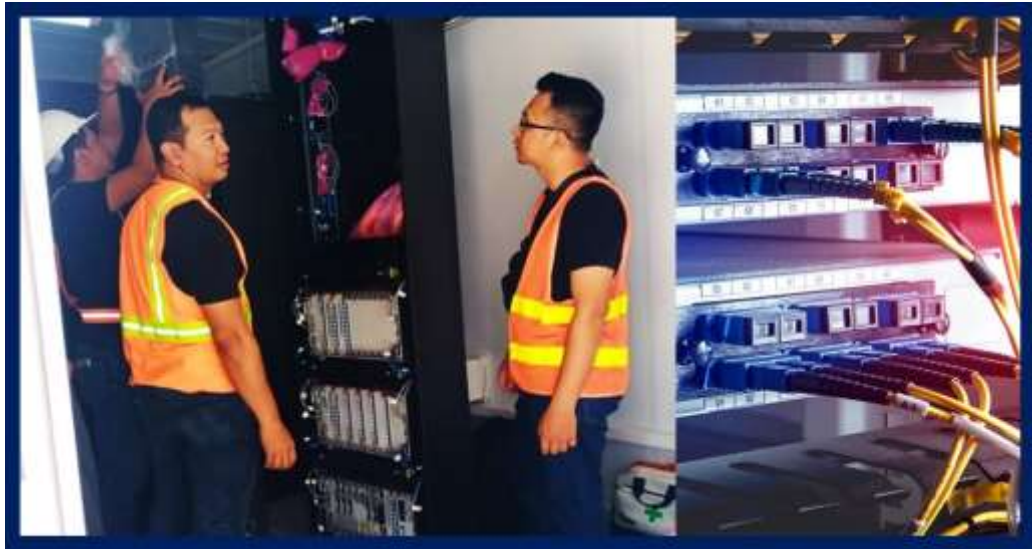
Gambar 5. Layanan Kolokasi Data ( Colocation ) Perseroan (Sumber: Internal Perseroan)
